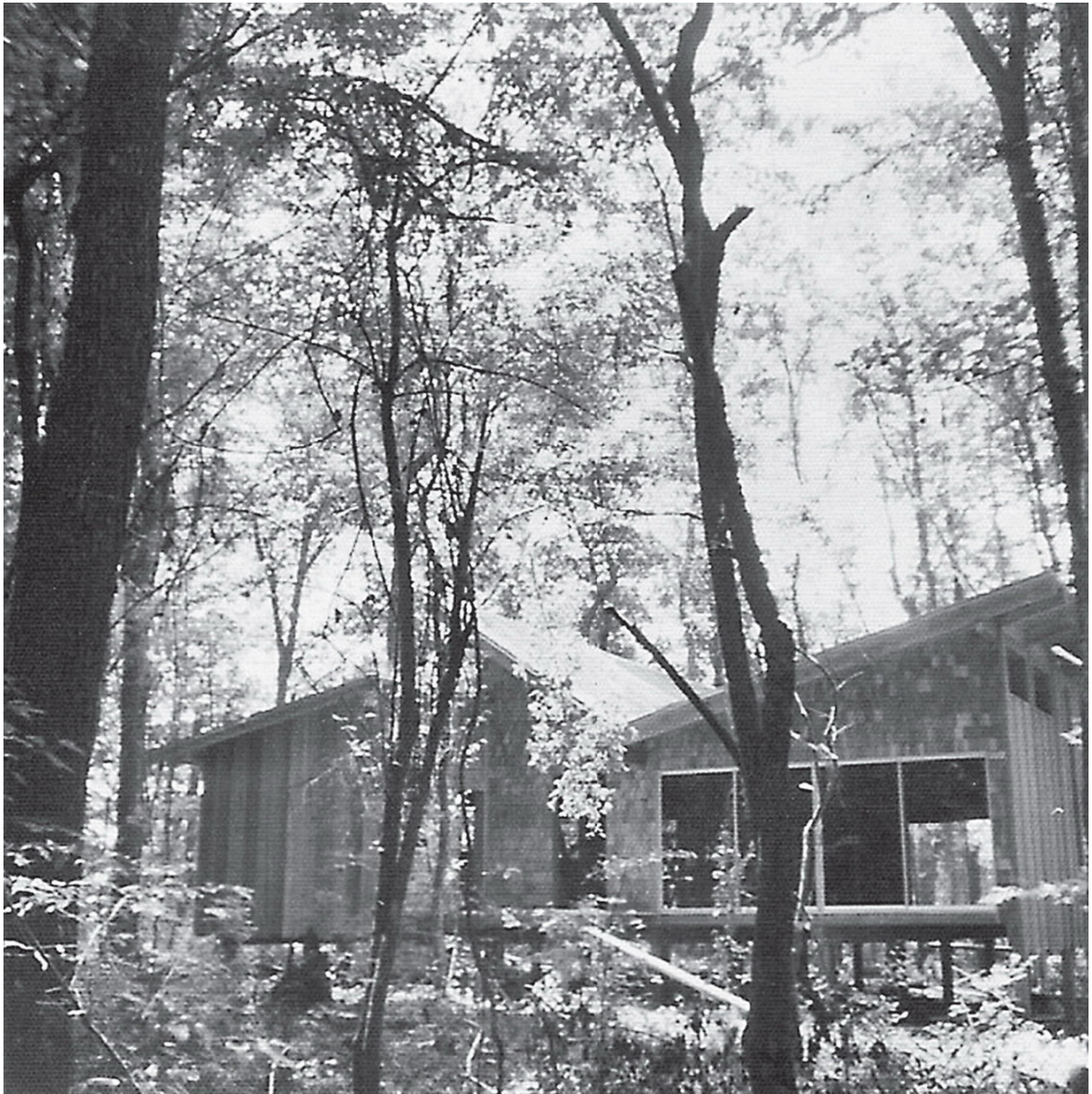
The Temple of the Universe, with its dynamic butterfly roof, under construction, 1975.
